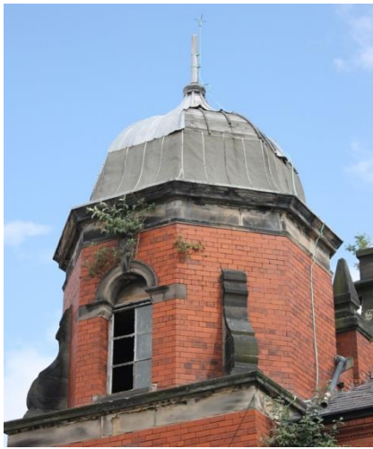
A disused church in Liverpool. The lead has been almost completely stripped. Amazingly the lightning conductor is still in place... for now!
