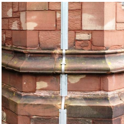
This lightning conductor is fitted with a protective sheath.
